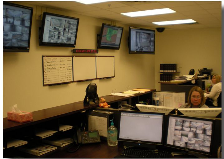
Pictured is the video surveillance monitoring station at Leon County, Florida, Public Schools.
